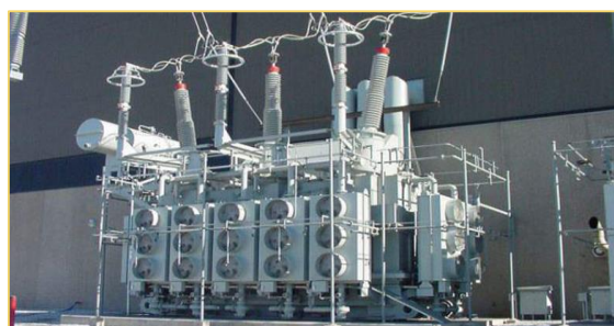
Figure 8 power generation plant
