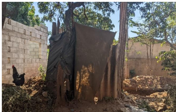
Figure 2: Insert pit latrine without slab in Kabanana
